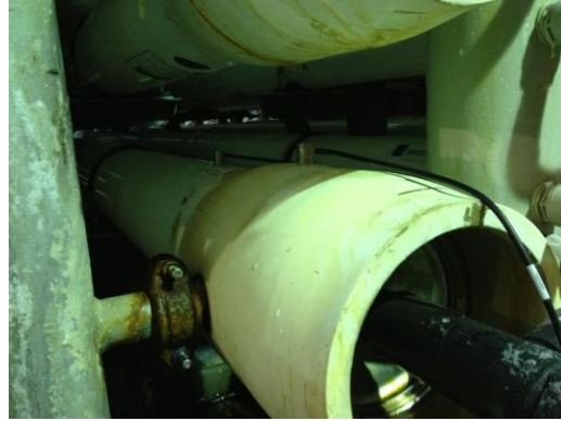
AE sensors during monitoring of Reverse-Osmosis FRP pressure vessel
